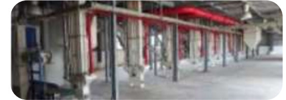
Rice milling facility
